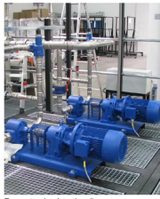
Pumps to circulate the oil
